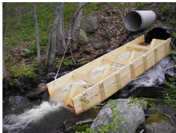
Improperly installed culverts can impede movement and restrict habitat connectivity for many aquatic ecosystems. In this case, a fish ladder may allow some species to traverse the barrier. © Department of Marine Resources
